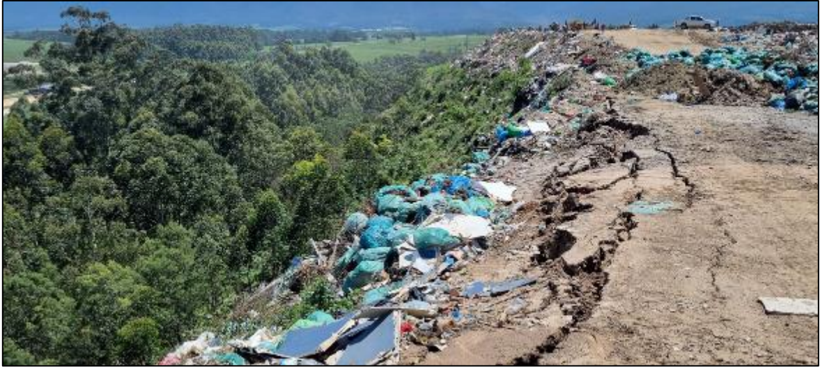
Figure 5: Slumping evident on the steep western face of the landfill.
